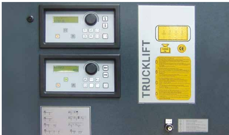
Central control and programming unit with two displays.
